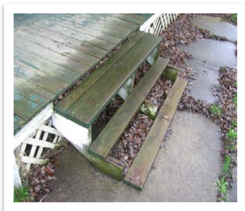
Damaged/missing treads and risers.
