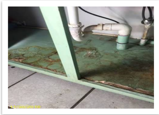
Chemical residue left under a sink.
