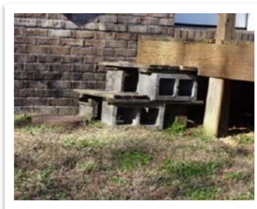
Unacceptable use of materials.
