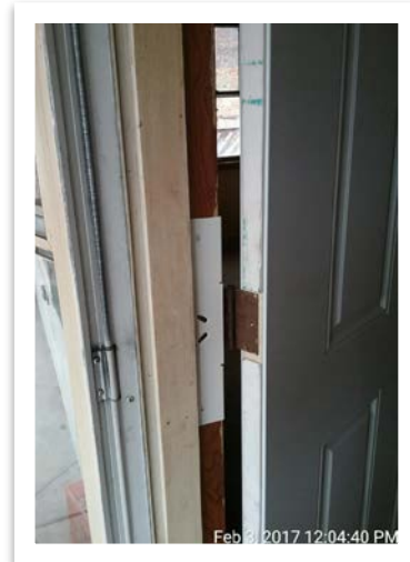
Photo showing door hinge protection product installed.
