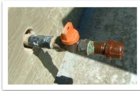
Gas line shut off and capped correctly.
