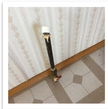
Incorrect type of gas line cap.
