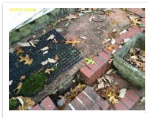
Bricks used for a riser are missing creating a trip hazard.
