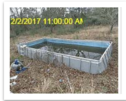
Pool must be drained and dismantled.
