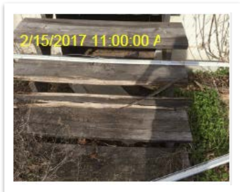
Damaged treads and risers.
