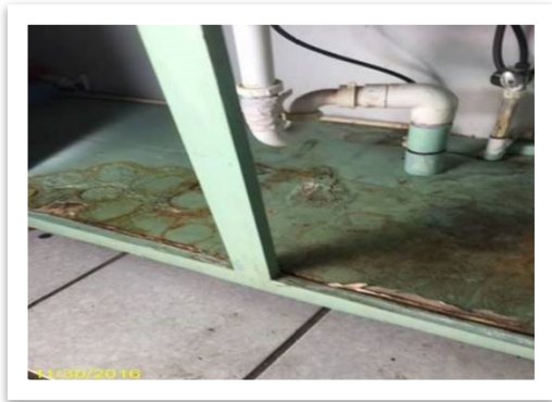
Chemical residue left under a sink.
