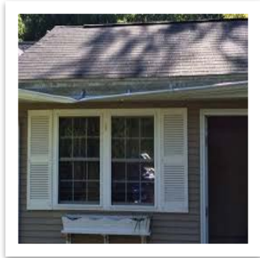
Section of gutter needs repair.
